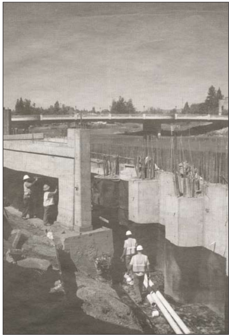
Contractors install a drainage system for the future river promenade in front of the Napa Mill earlier this year. Register file photo
