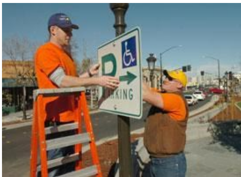
Maintenance workers Kris Franklin, left, and Jason Calkins install a parking sign on South J Street in Livermore's new downtown.
